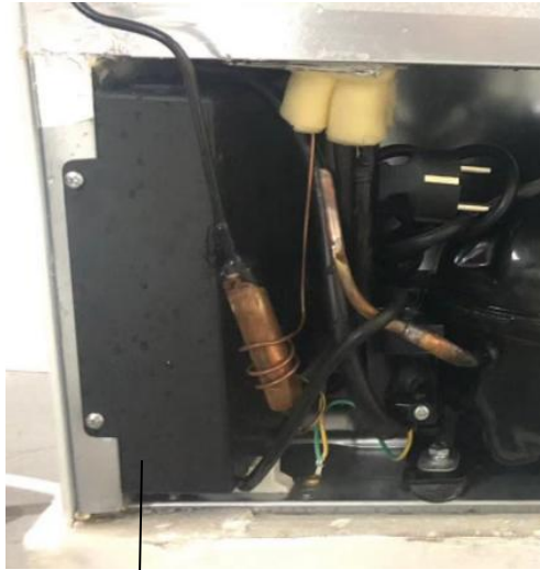
Control board epair from the lower left of the back
